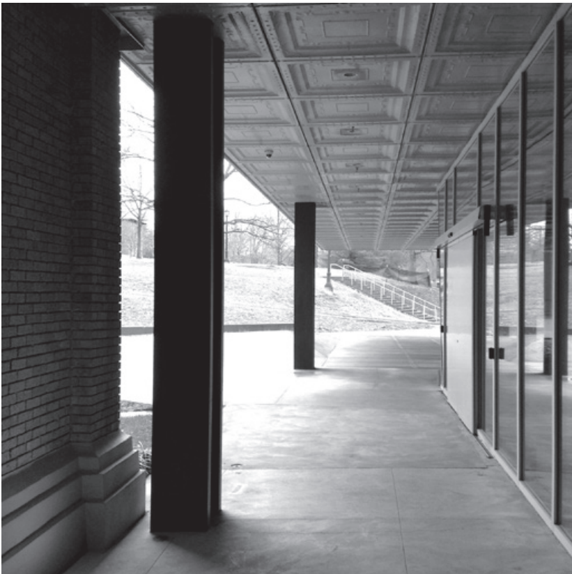
Figure 12.10. The exterior steel columns in OMA's Milstein Hall at Cornell act as thermal bridges by penetrating through the insulated soffit.
